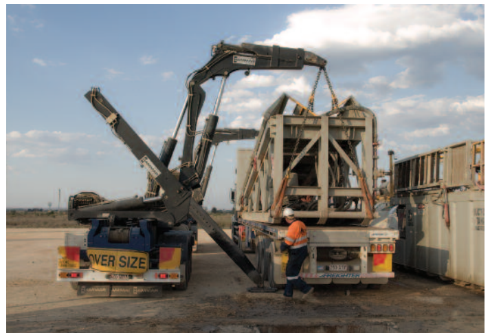
Hammar Rig Lifter has many uses in the field, note well head in foreground
